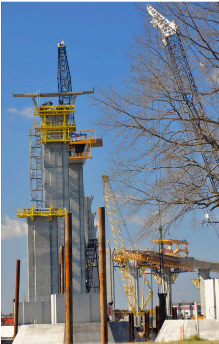
Progress on the new South Norfolk Bridge continues. It is anticipated to be open to drivers by late spring/early summer.
